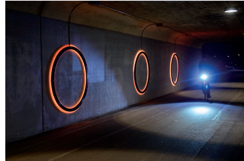
Adaptive tunnel lighting in Gladsaxe Municipality, Greater Copenhagen region. © Cycle Superhighways
